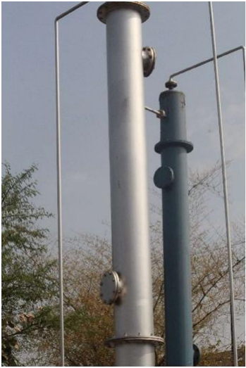
Scrubber Tower at RKDF
