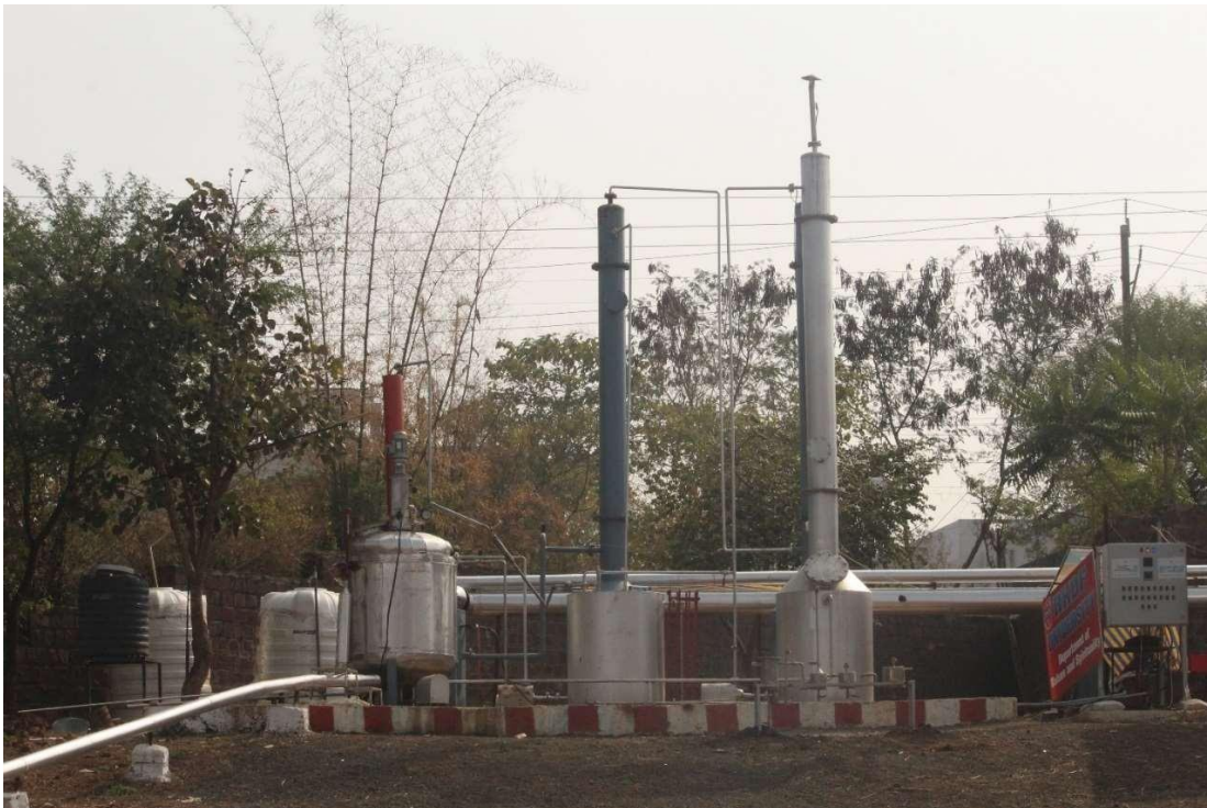
Figure 1: CCS Plant at RKDF University
