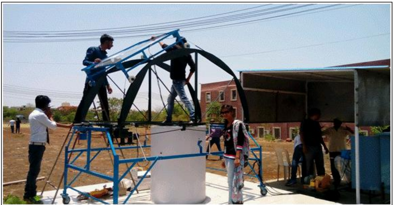
Figure: 2. Installation of the solar thermal storage and solar tracker unit at RKDF university
