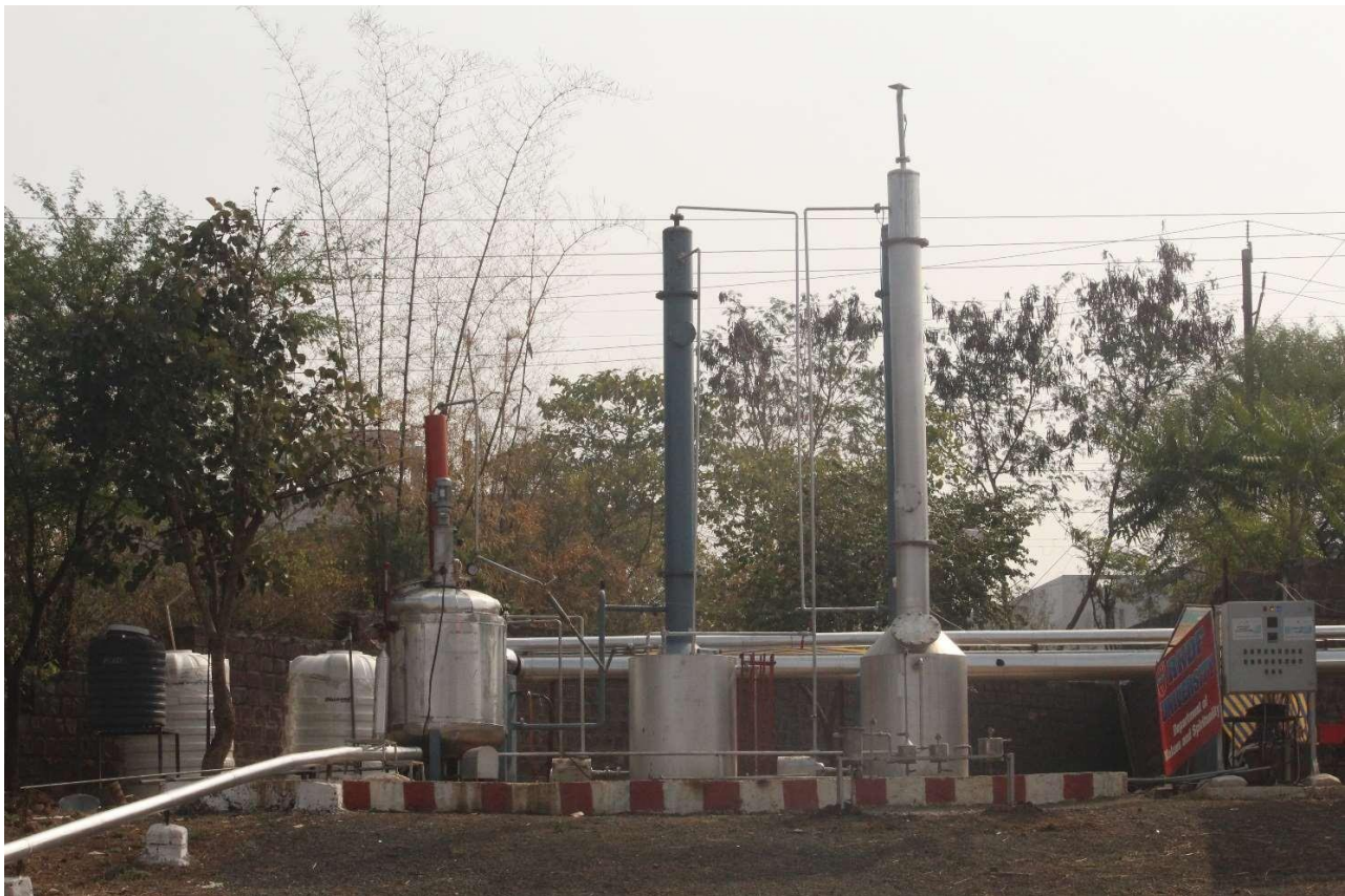
Figure 1: CCS Plant at RKDF University
