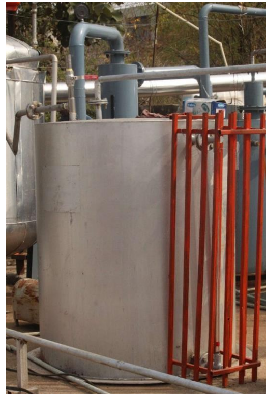
Intermediate Tank at RKDF
