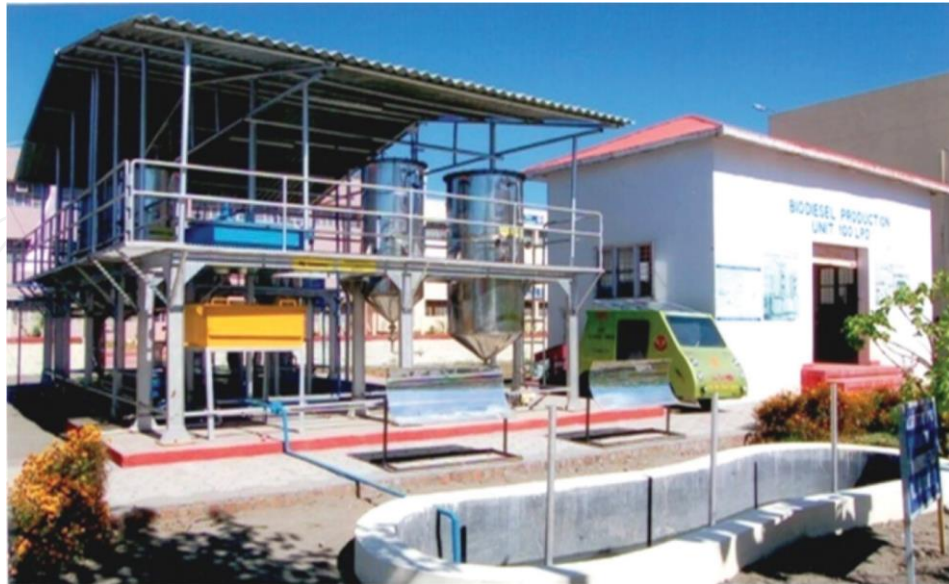
Figure- 2 CO 2 capture & sequestration plant (CO 2 & steam source—oil fired baby boiler).
