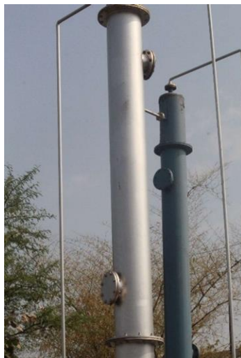
Scrubber Tower at RKDF
