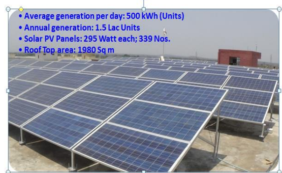
100 kW Roof Mounted Solar PV Plant at RKDF University
